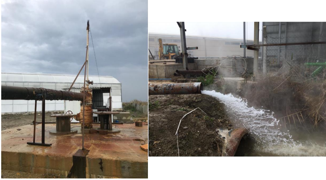
Figure 4.1. PS-1 well and well discharge through pipe in Akköy geothermal field
